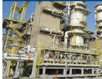
Gas Pre-Treatment and Nitrogen Rejection Units
