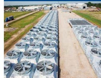
Air Cooled Heat Exchangers
