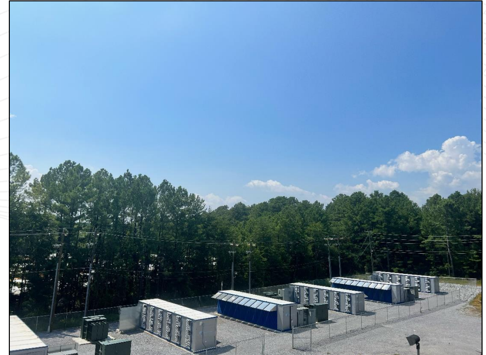
DGHI's Proposed Tier 3 Data Center Conversion Site
