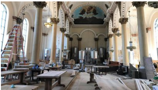
The conversion of old St. Michael's church into a brewery has been underway for months. (Baltimore Sun)
