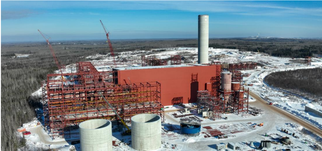
Exhibit 25: Construction Progress at Mesabi Metallics' Pellet Plant and Processing Facilities. Source: Mesabi Metallics
