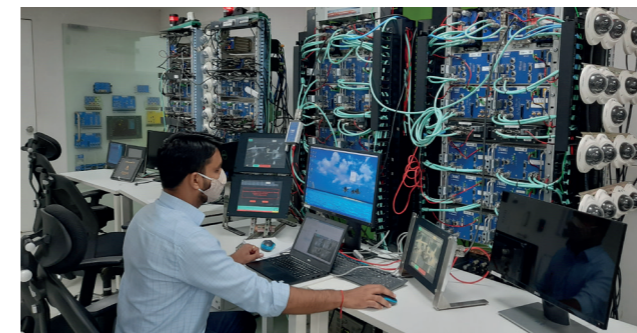
3 4 Bombardier's Channi and Atladara site in Vadodara will deliver Control Monitoring System
