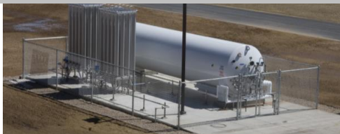
Liquid oxygen system for ozone generation (Duchense, UT)
