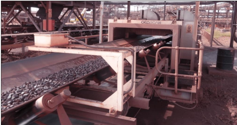
Exhibit 7: Conveyor-Based Sensor Ore Sorting System. Source: Company Website
