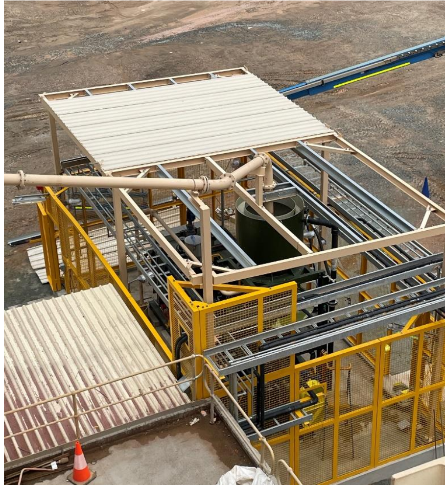
(Figure 6: Acacia gold-recovery reactor with guards and roof sheeting undergoing final stages of installation.)
